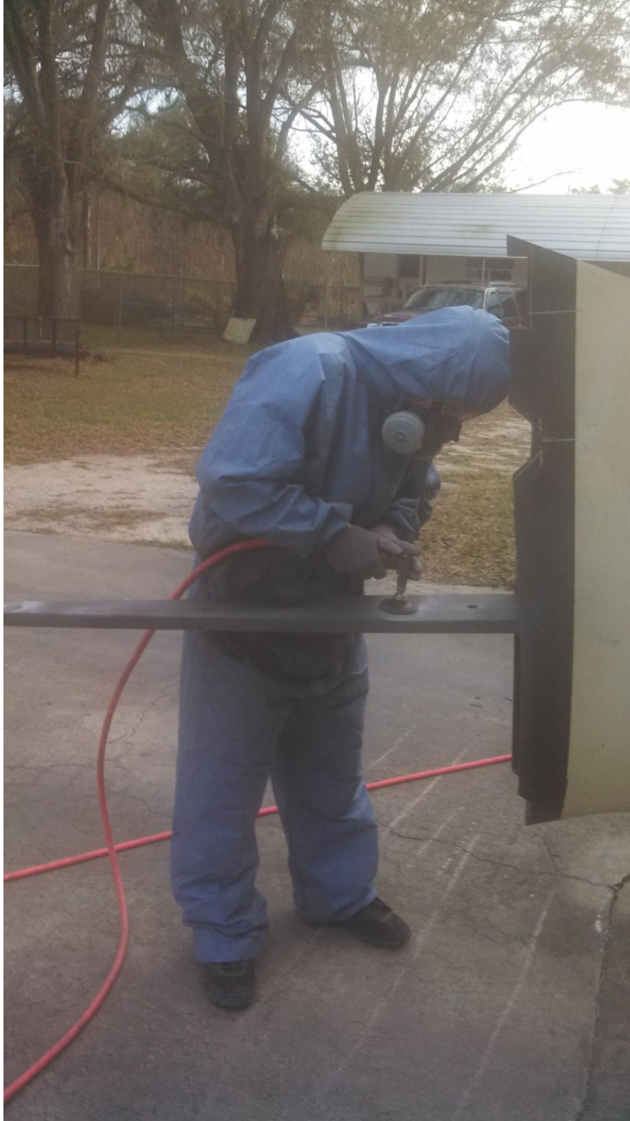
Figure 2 shows the builder properly protected.
